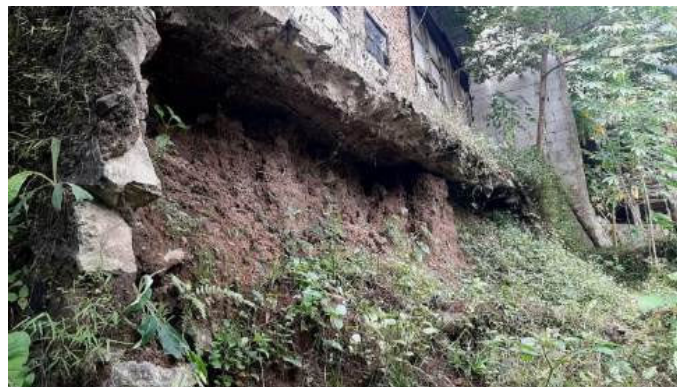
Figure 11. Landslide around the settlement area in Rongga district.
